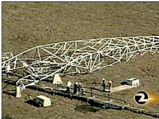
PG&E Redwood City wetlands December 26, 2006 High winds & defect
