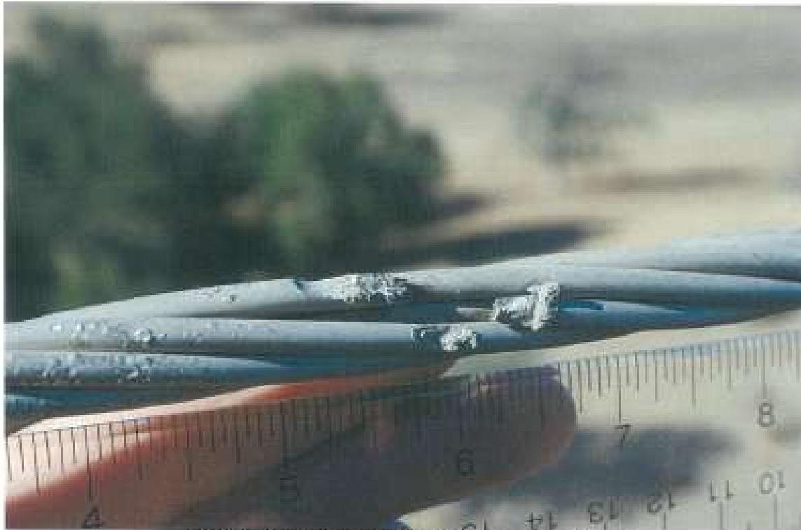
P-64 MG Close-up view of damage to lines
